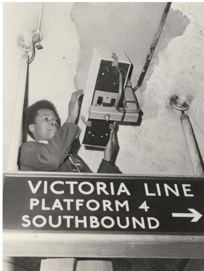
Fig. 11 Photograph from London Transport Museum of a CCTV camera being installed on Victoria line on the London Underground in the 70s.
