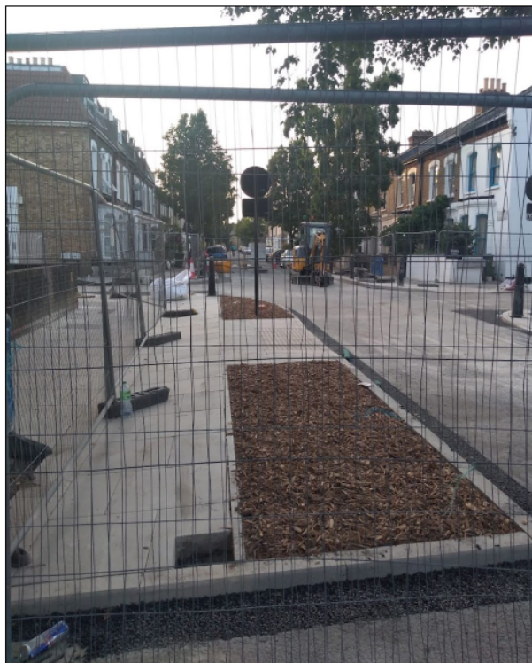
Figure 35: Maintenance works observed at the Rattray Road/Jelf Road modal filter (Author's own, 2022)
