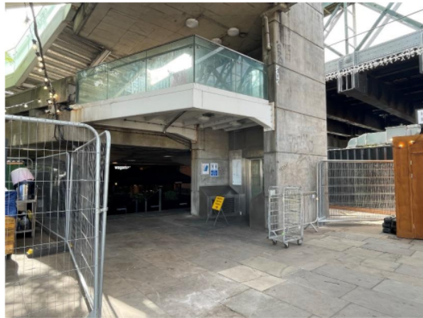
Photo 10 - Unwelcoming: Accessible options are available in South Bank, but some, such as this elevator that is provided for the access to the Festival Terrace and Golden Jubilee Bridges, are highly vandalized with graffiti, looks dirty and smells bad. The lack of cleanliness leads to people avoiding using this facility.
