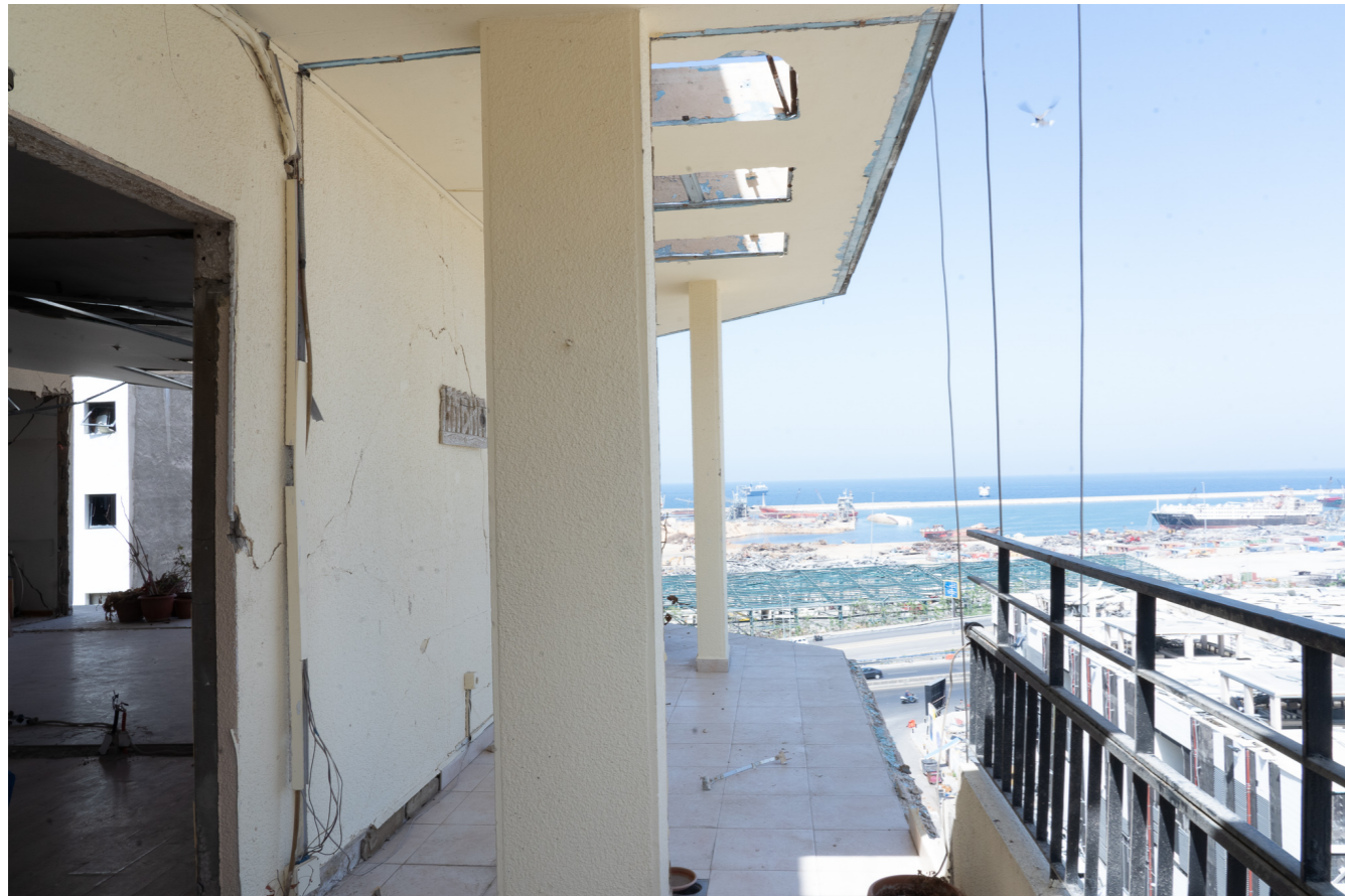
Image 004: Flat Damaged by Blast in Medawer (source: Lynn Malas, Nusaned)
