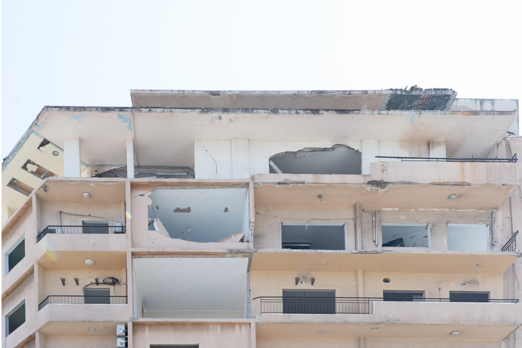
Image 006: Façade of Damaged Building in Medawer Area
