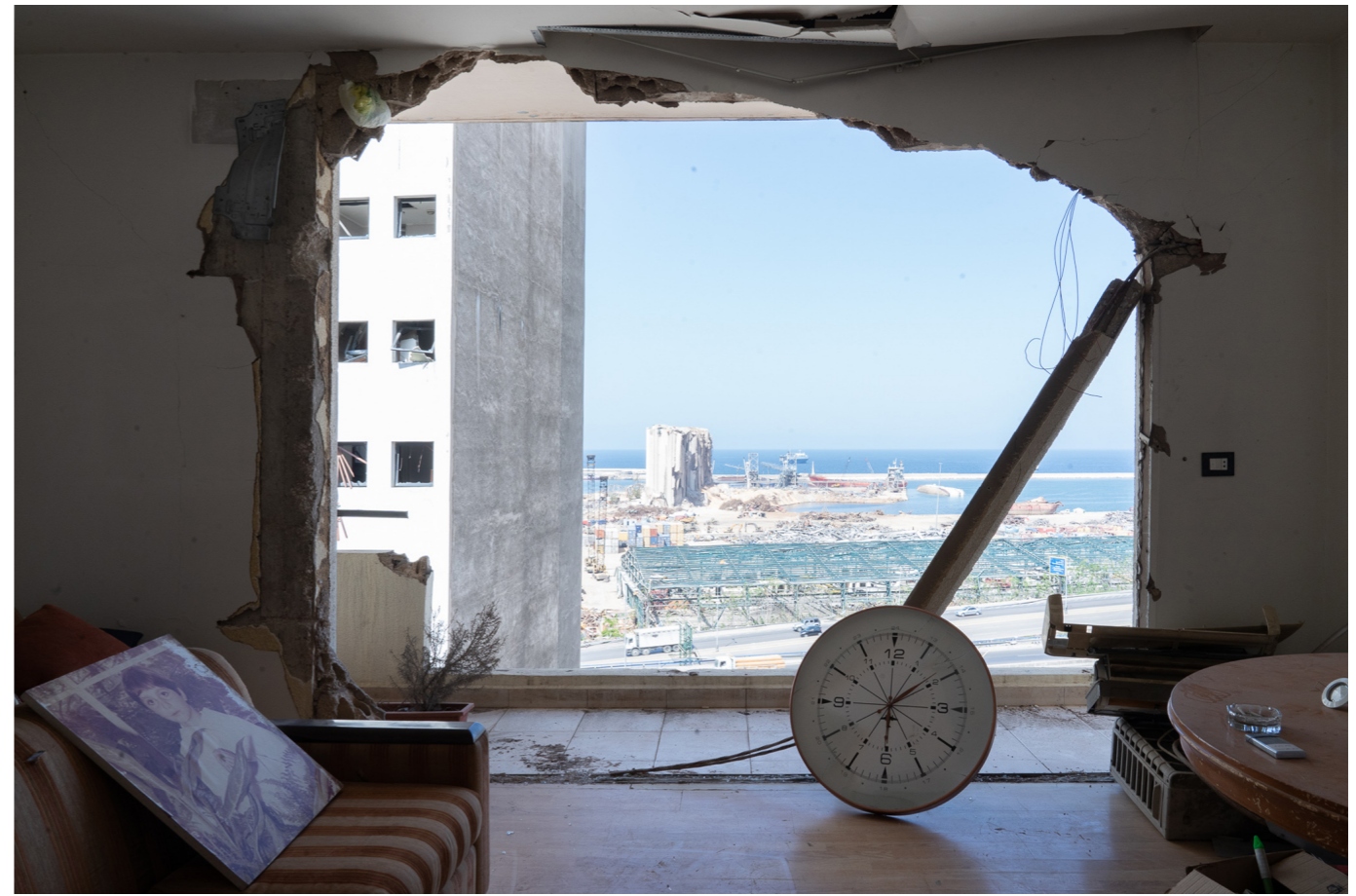
Image 005: Flat Damaged by Blast in Medawer (source: Lynn Malas, Nusaned)
