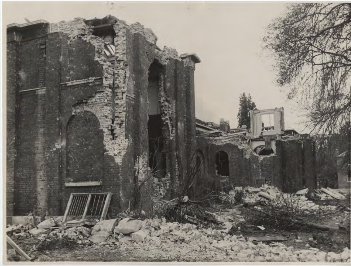
Figure 21: Bomb Damage to the Mausoleum and West façade (20 July 1944, photograph) © Dulwich College.
