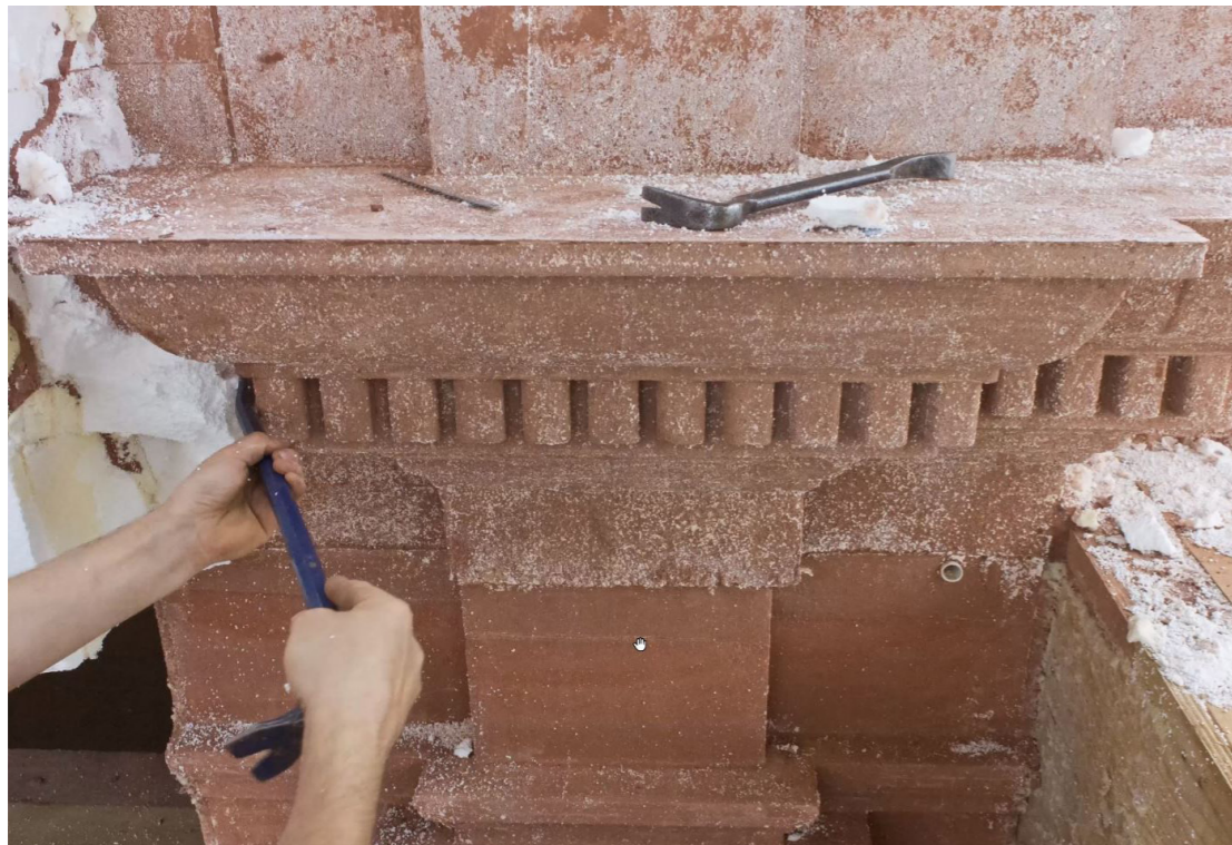
Fig. C11 (left): Remove of the polystyrene mould after the cast, Aria building. Fig. C12 (right): The drawing shows the two proposed construction methods for Aria Building. The polystyrene mould cast was cheaper than the precast concrete method.
