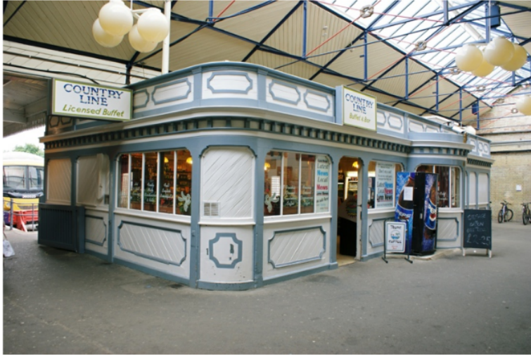
Figure 20 The Country Line Buffet Bar at Grade II listed King's Lynn Station. Under GTR, it too has received a similar heritage restoration in 2016 focused on finding sustainable reuse for non-operational parts of the listed structure.
