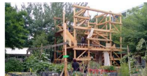
Figure 29 Experimental playground built from recycled timber by community volunteers - a form of community co-production alongside food growing
