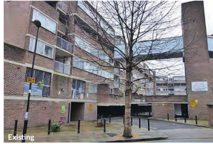
Fig 45: Security problems as a result of the public access, basement garages and the raised walkways.
