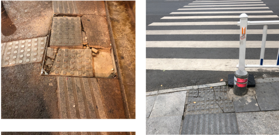
Figure 17 and 18. Cracked tactile paving (Author, 2019).
