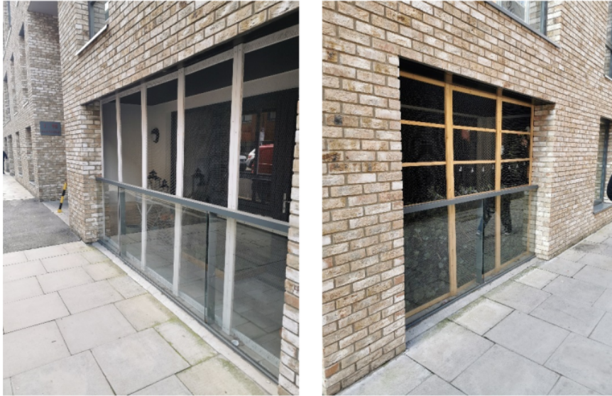
Figure 21: Some inset balconies along Wharf Road have been fortified with chicken wire mesh
